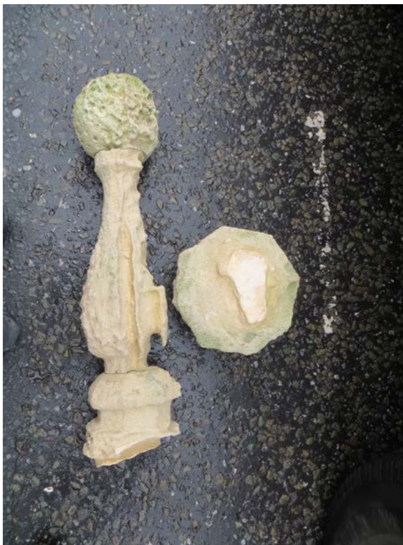
Dangerous rooftop objects temporarily removed
